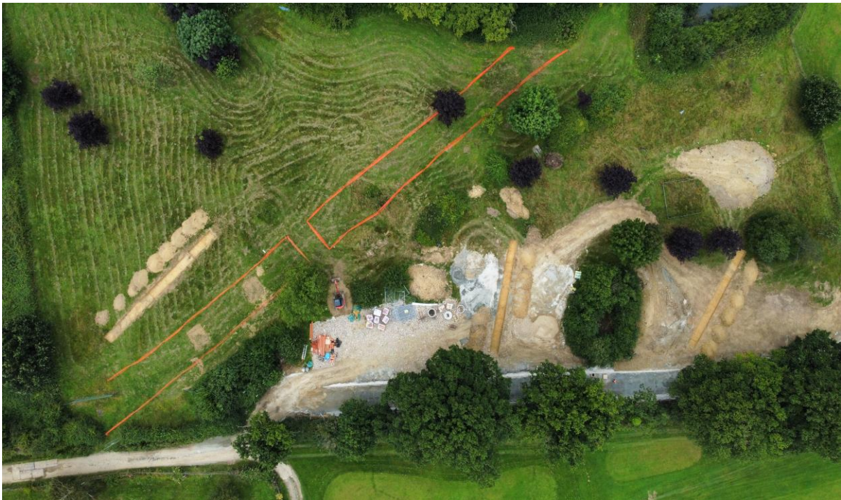
Plate 2 Aerial view of the three trenches excavated within the site (note: safety fencing providing protective for the existing gas main)
